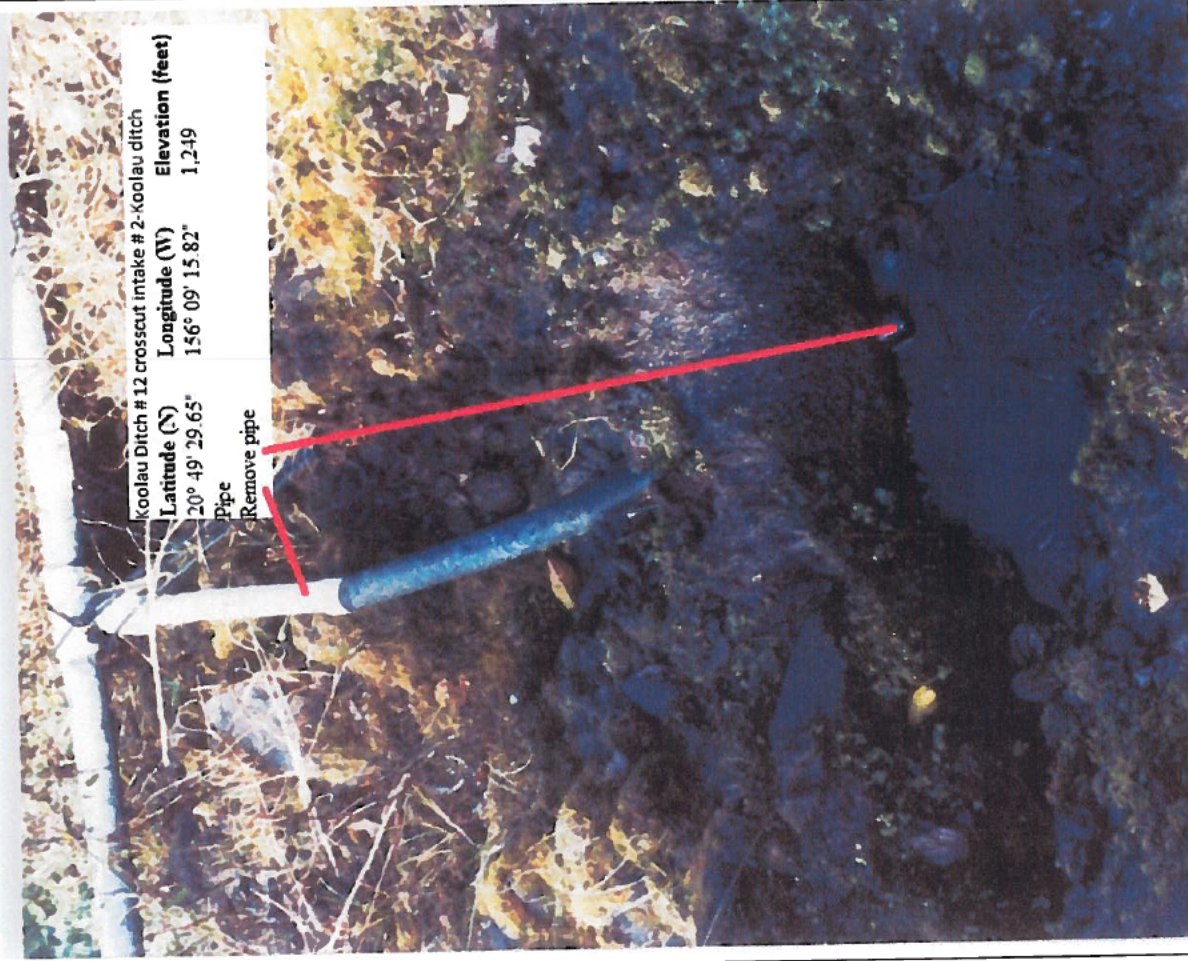
Photo 15: Number 12 crosscut intake at Koolau Ditch #2 of 5 (K-24b) Pipe shown was removed in 2007.
