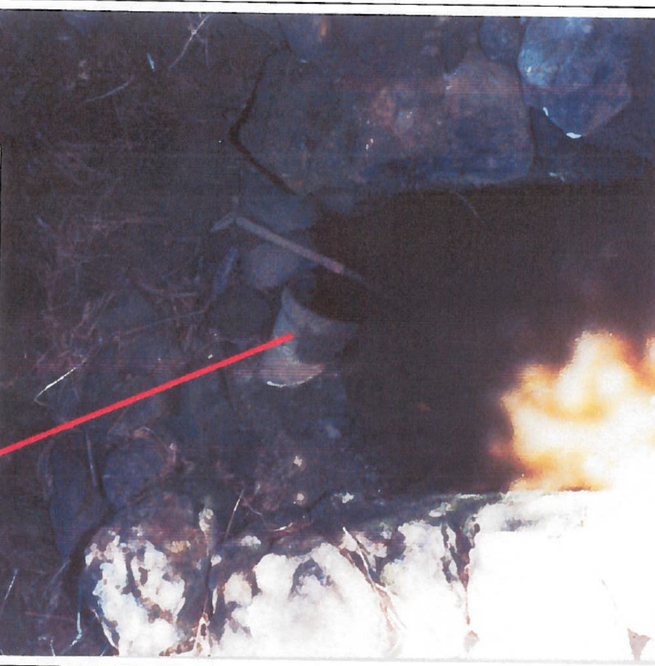
Photo 2: 6-inch Kualani (East Waiokamilo) aluminum pipe at Koolau Ditch (K-22a) Pipe shown was removed in 2007.
