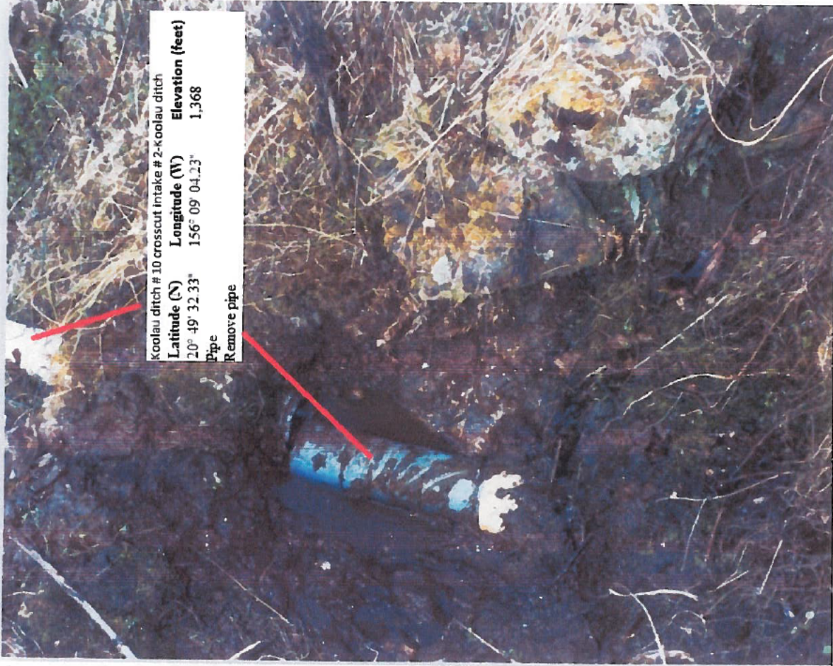
Photo 4: Number 10 crosscut intake at Koolau Ditch, #2 of 6 (K-22c) Pipe shown was removed in 2007.
